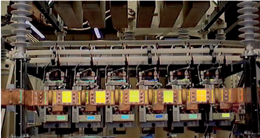
Fig. 3: Vibration modes on the semiconductor modules on the front of the converter.
