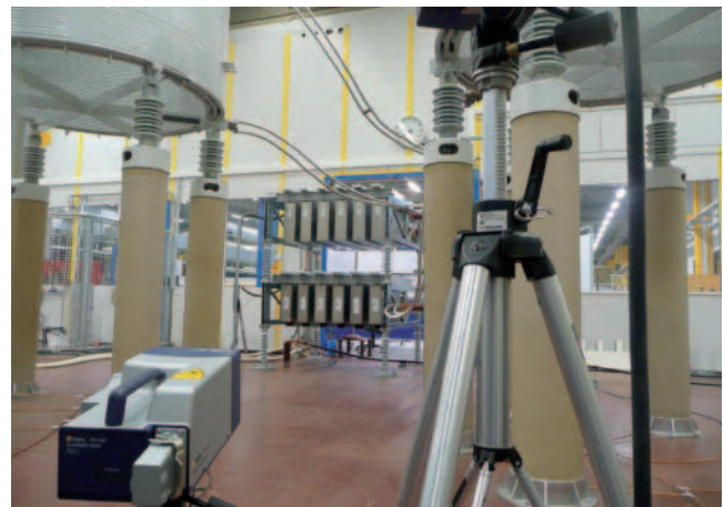
Fig. 2: HVDC test facility, scan heads set-up for testing the rear side.
